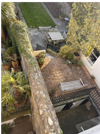
Existing condition looking down on party wall from number 11 to number 10. There is nowhere for vegetation shown in the imagery to grow (2 in image below).
